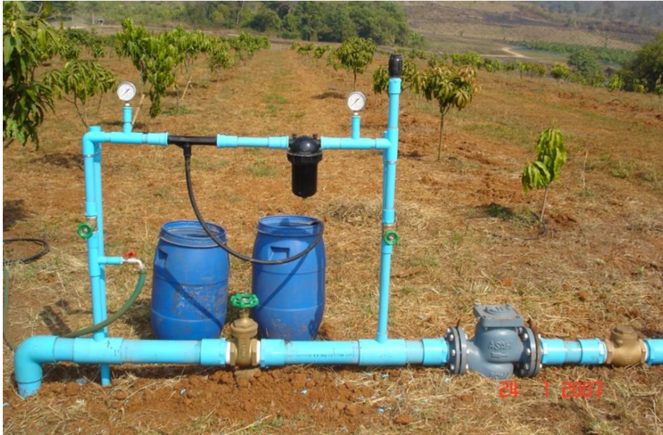
Figure 11: Sub-head station with fertilizer injection and secondary filter (picture: S. Chotivan)
