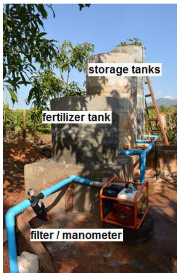
Figure 20: Head station with storage tanks
