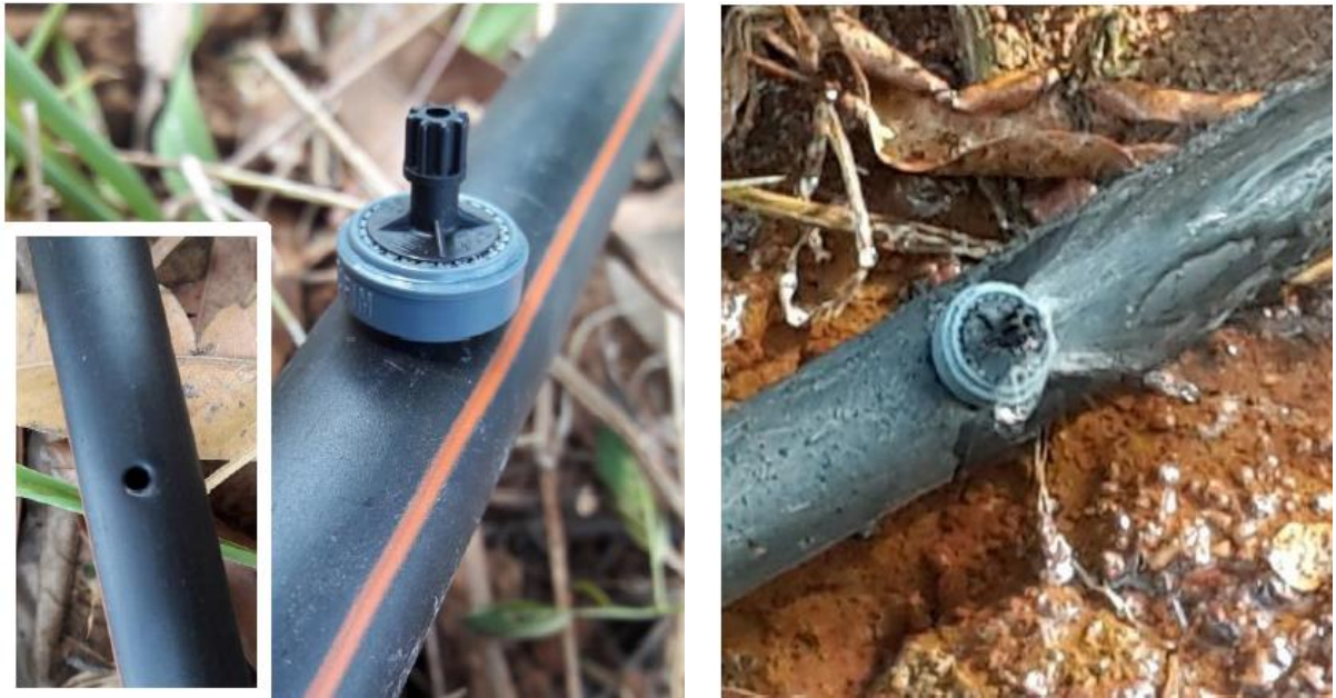
Figure 26: Left: Well-installed plug-on dripper; no leakage – the exact amount of water is delivered to the plant. Right: Leaking dripper due to sub-optimal pipe material used.
